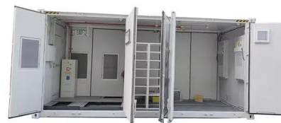
1075KW HH ESS
