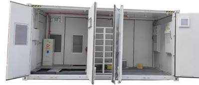
1075KW HH ESS
