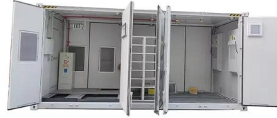
1075KW HH ESS
