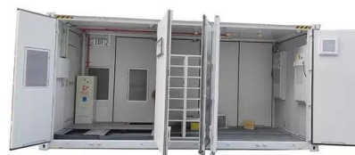
1075KW HH ESS
