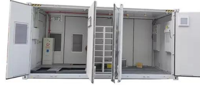
1075KW HH ESS
