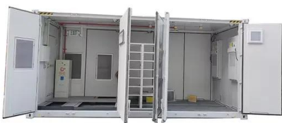
1075KW HH ESS
