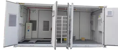
1075KW HH ESS
