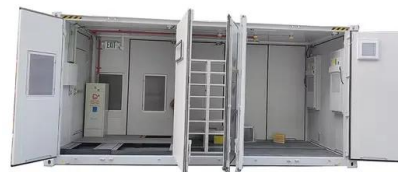
1075KW HH ESS
