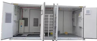
1075KW HH ESS
