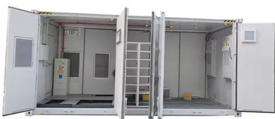
1075KW HH ESS
