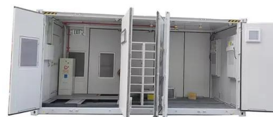
1075KW HH ESS
